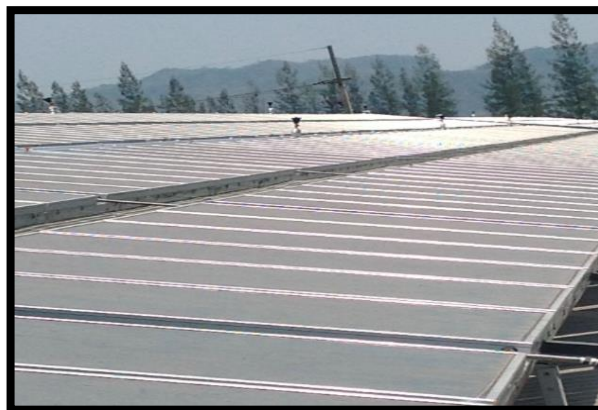
(b) The solar rooftop system for energy generation used on-farm
