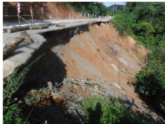
Figure 8. Show the area and nature of the failure of a slopes in Highway no. 108, section Mae Rid Bridge-Huai Ngu at km. 158+865 - km.158+923 RT.
