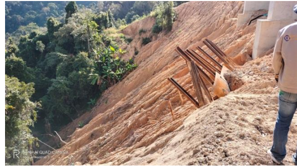
Figure 7. Show the area and nature of the failure of a slopes in Highway No.1263, section Khun Yuam - Pang Ung, at about 18+580 km LT.
